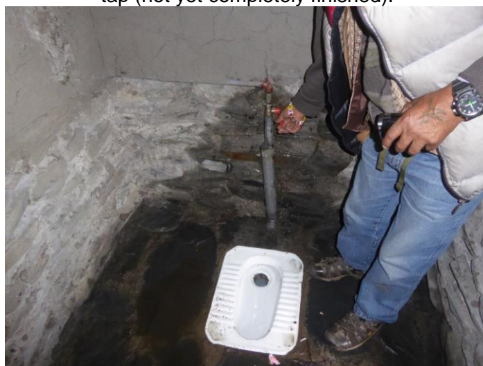
Water connection from inside, equipped with a simple tap (not yet completely finished).
