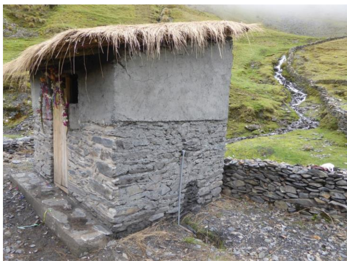
Water connection from outside.
